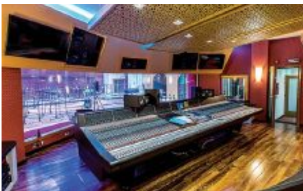
The control room for Katara's studio 1
